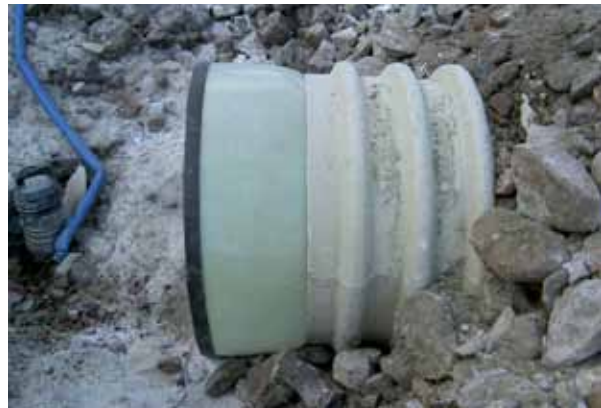
The lining expands at the ends of the culvert and stabilize the embankment.
