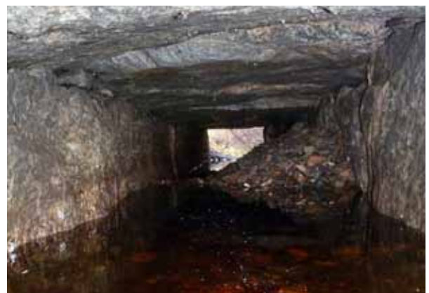
This is often the case in older stone culverts; the stones have separated and gravel and mud pours into the culvert.
