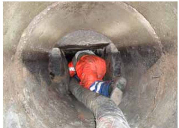
Effective cleaning of the culvert is the first step in order to achieve a perfect result.
