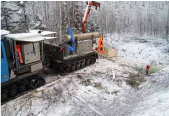
The installation equipment is transported on a tracked vehicle with low ground pressure. Refurbishment can thus be performed regardless of the tracks are closed or not.
